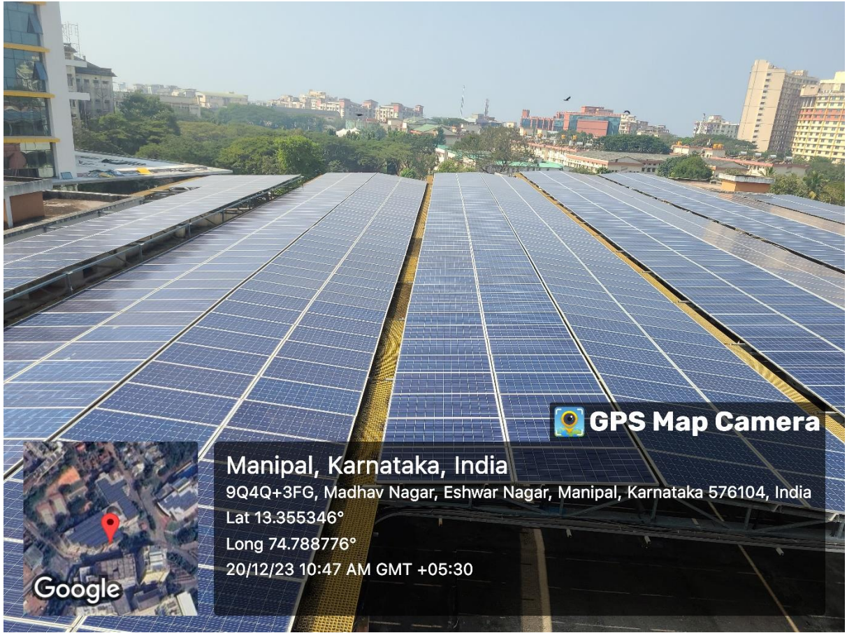
Solar Photo-Voltaic Panels
