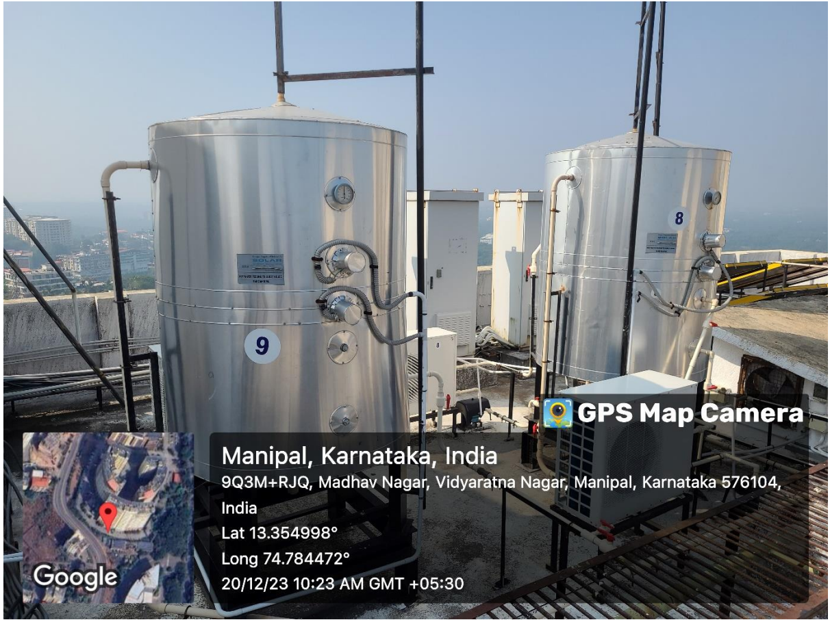
Solar Hot Water Systems
